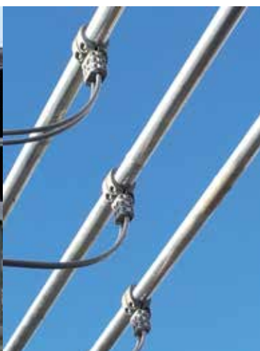
GPO 110/15 kV Jędrzychowice
